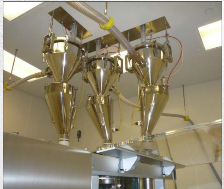
Continuous vacuum conveying of pharmaceutical powders to capsule filling machine.
